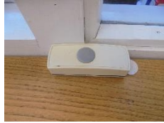
Bell inaccessible and no signage
